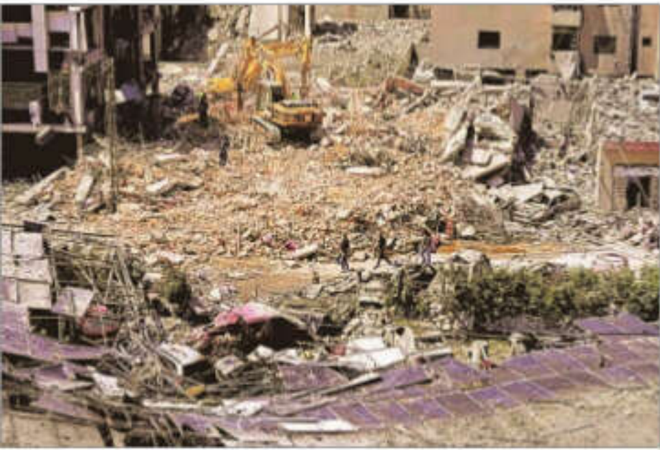
Rescue workers use excavators, as they search for victims under the rubble of a building that was hit in an Israeli airstrike in the southern port city of Tyre. REUTERS
